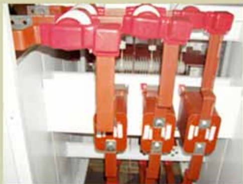
Custom 15 KV Switch and Transition to Transformer
