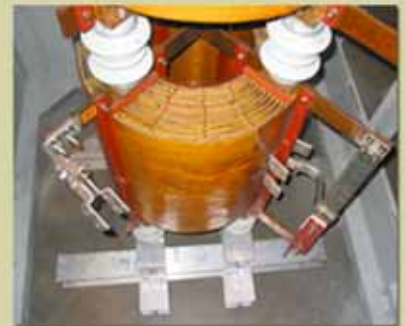
15 KV, 1600 A Current Limiting Reactor Assembly
