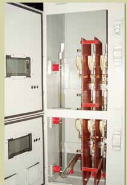
15 KV Duplex Switch
